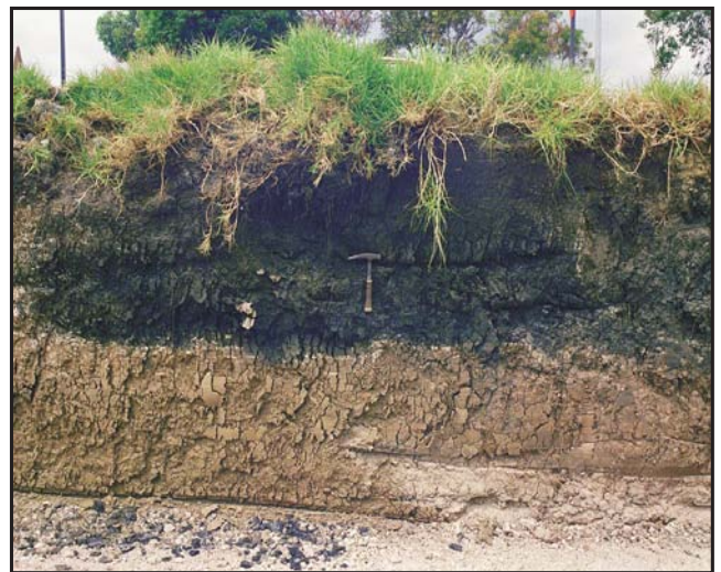
A black cracking clay soil overlying the Keswick Clay (both extremely reactive materials) exposed in an excavation at Modbury. (Photo 43664)
