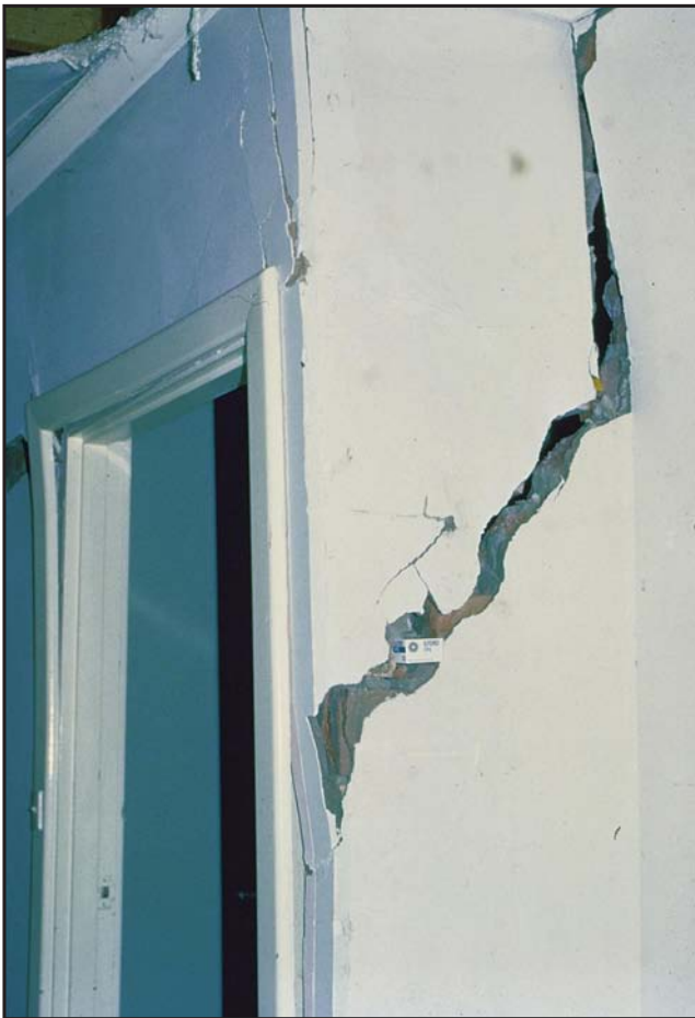
Severe cracking in a domestic house internal wall in the Athelstone Park area caused by differential heave of a black earth soil and the underlying Keswick Clay. (Photo 42051)
