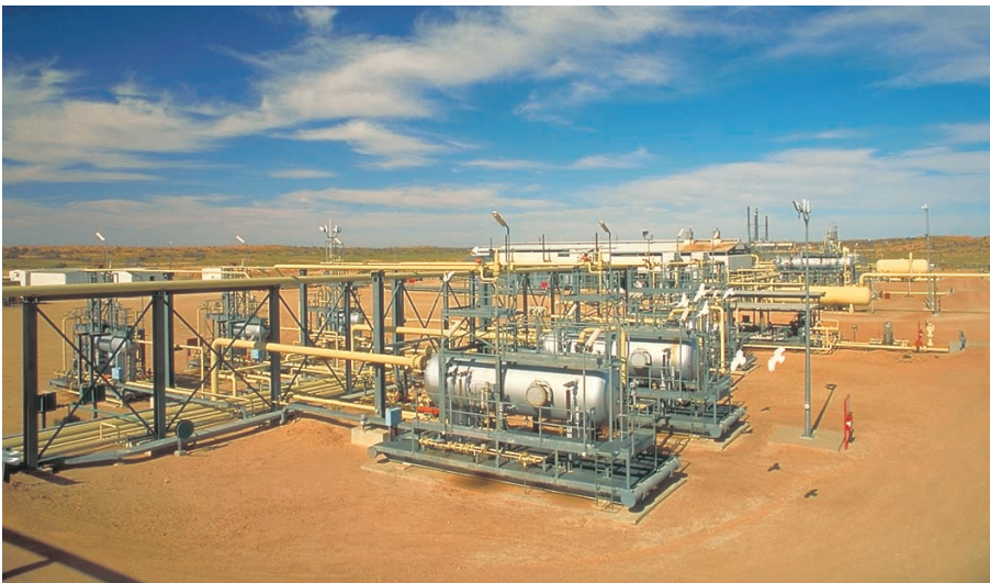
Tirrawarra oilfield satellite, Cooper Basin (Photo 43356)
